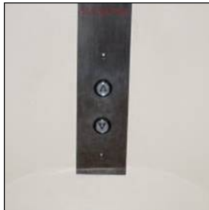
Figure 24. Up and down elevator buttons.
